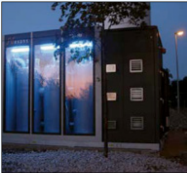
Test installation of superconducting fault current limiters. Nexans uses superconducting wires from American Superconductor.
