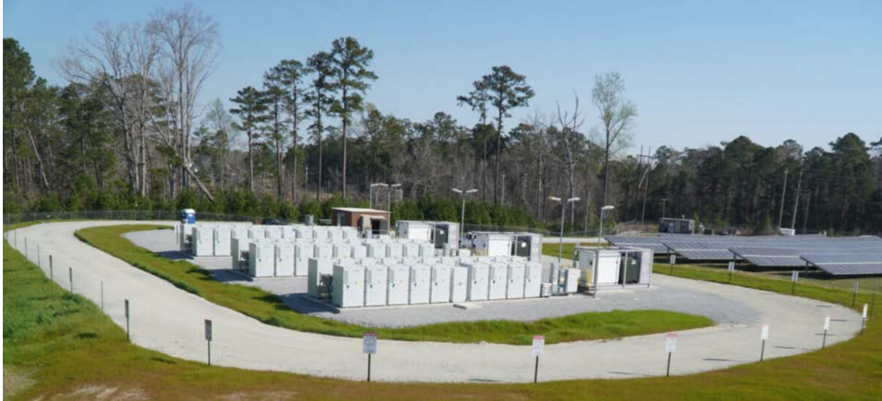
Figure 11: Energy Storage System at Camp Lejeune
