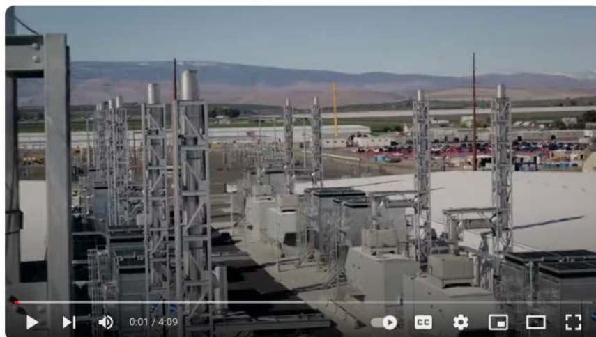
Figure 1: “Microsoft Reveals its Massive Data Center (Full Tour)”
