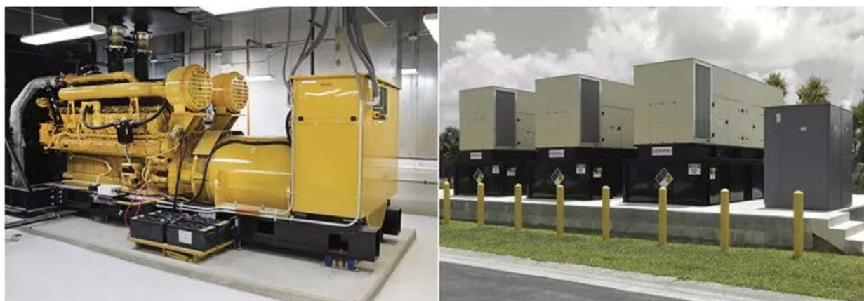
Figure 17: Example of an Indoor (Left) and Outdoor (Right) Generator Installation
