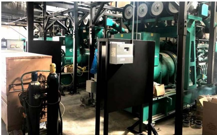
Figure 13: MCAS Miramar Microgrid Power Plant 480v and 12kV Switchgear and Generators
