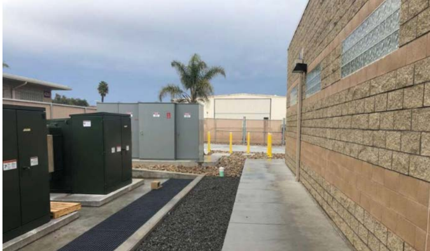
Figure 12: MCAS Miramar Microgrid Power Plant
